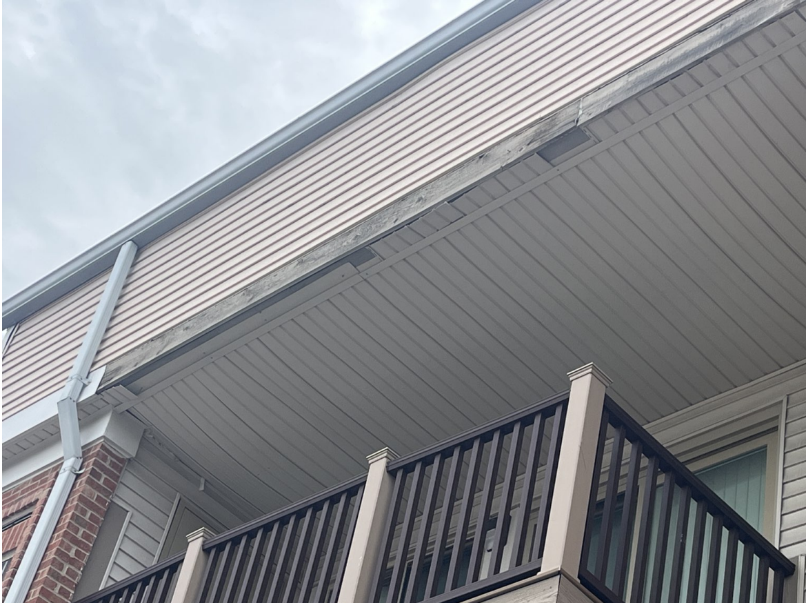
Soffit missed and sagging above deck. Sagging not show in picture. Aluminum trim to be fabricated and installed.
