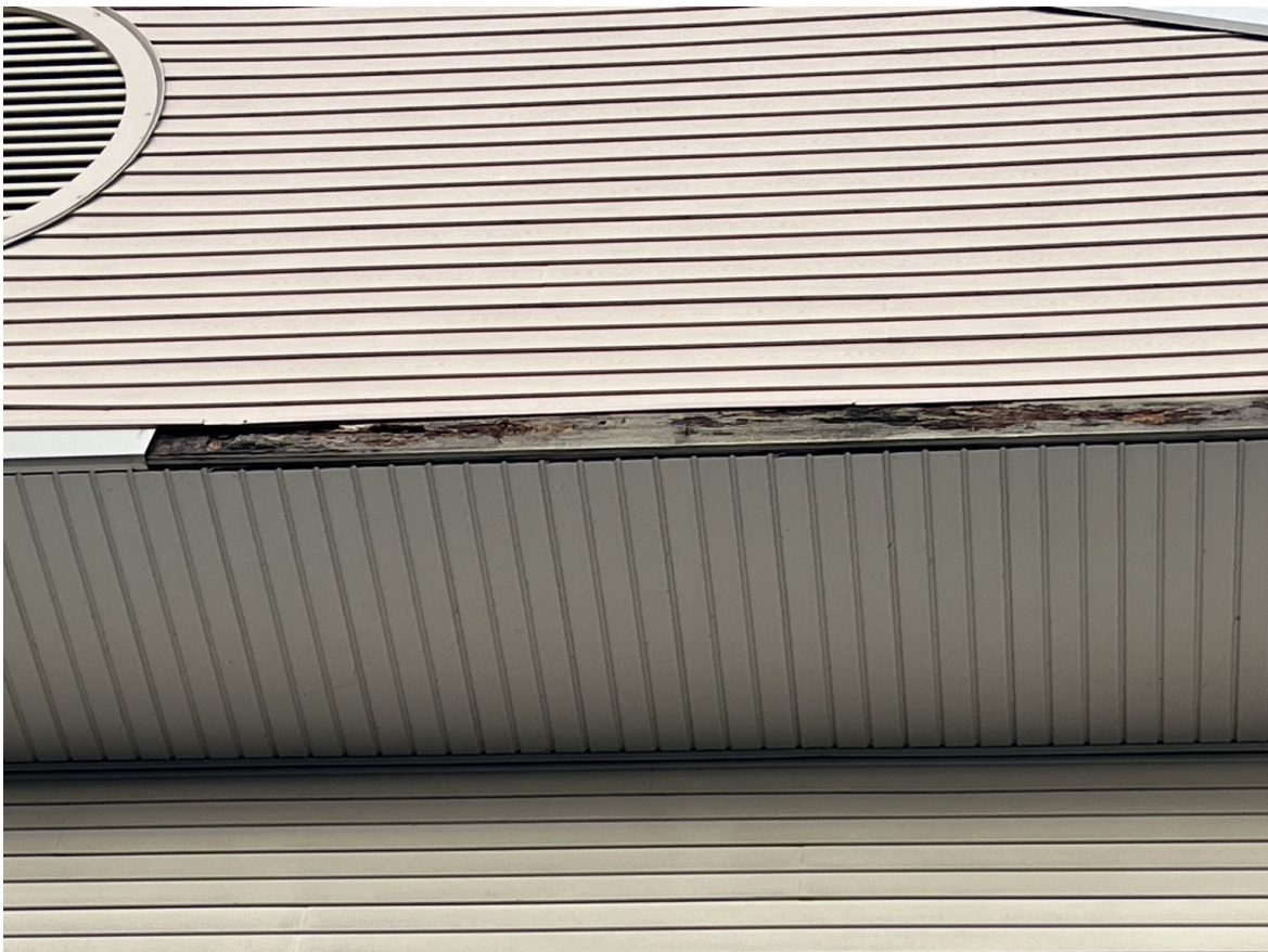
Water damage to fascia boards
