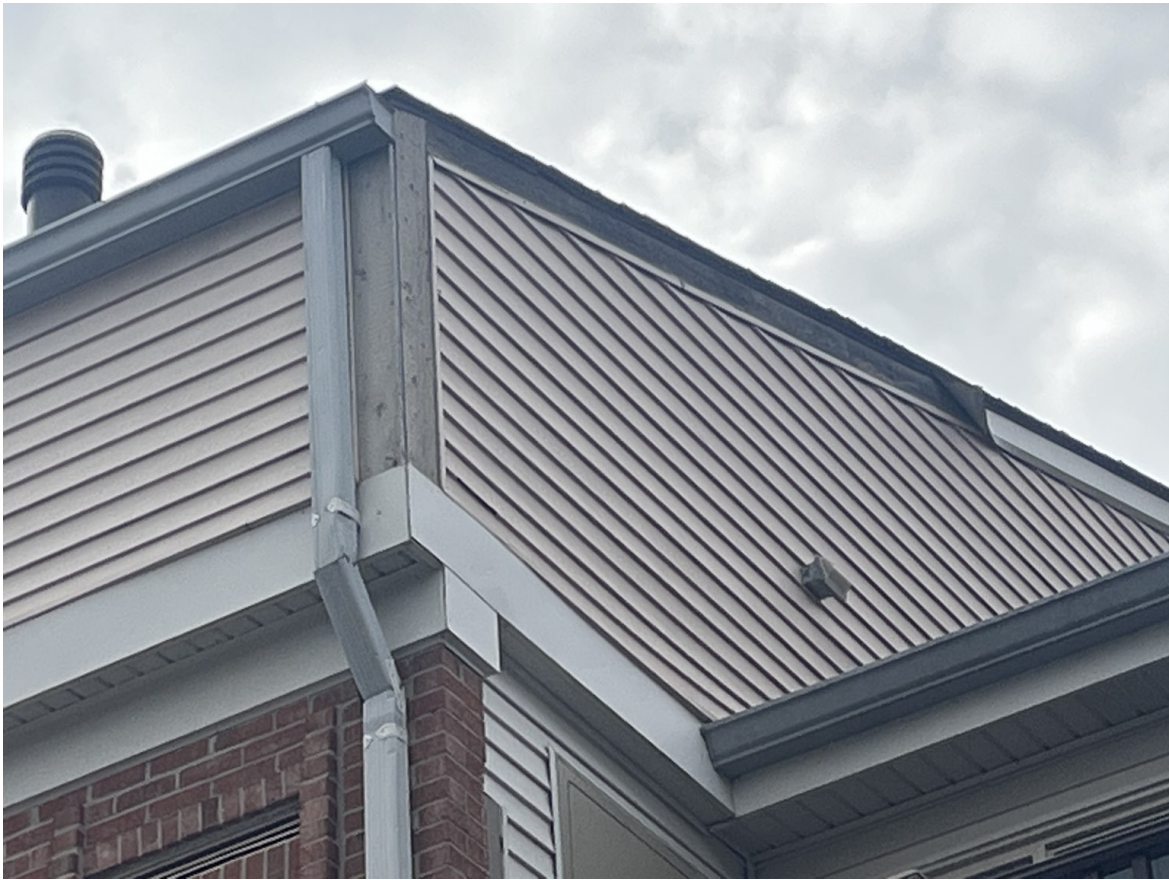
Some examples of aluminum trim to be replaced.
