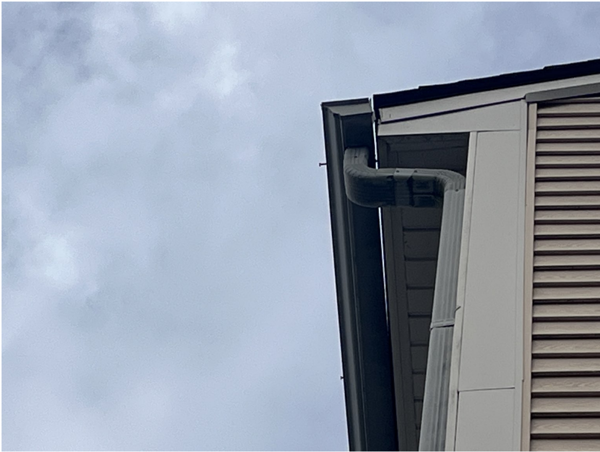
Example of gutters needing to be reattached at fascia.
