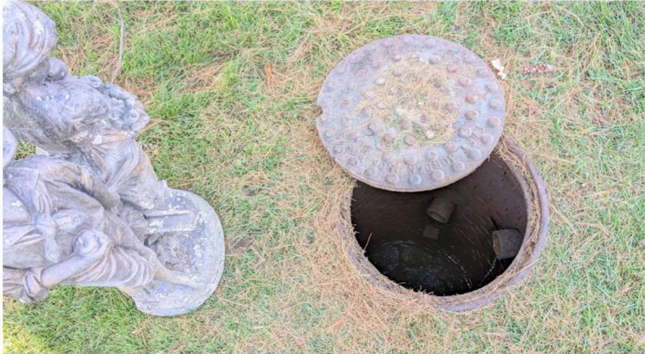
Figure 2: Flow from 31660 Linden Ave into Manhole LPS-2
