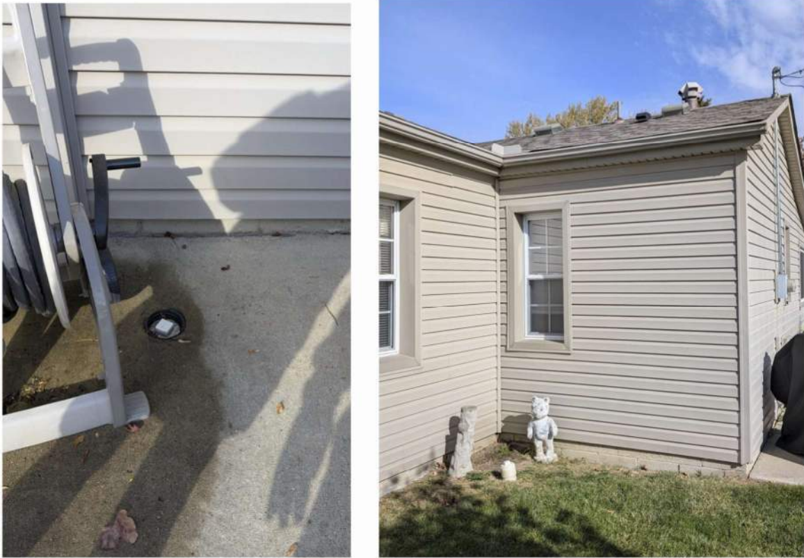
Figure 3: Two cleanouts at 31660 Linden Ave
