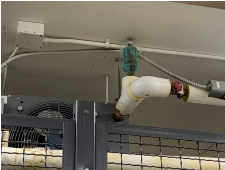
Photo 9: Hot Water Heating Air Vent-Note decolorization
