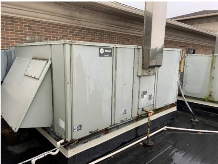
Photo 7: Rooftop Unit RTU-5
