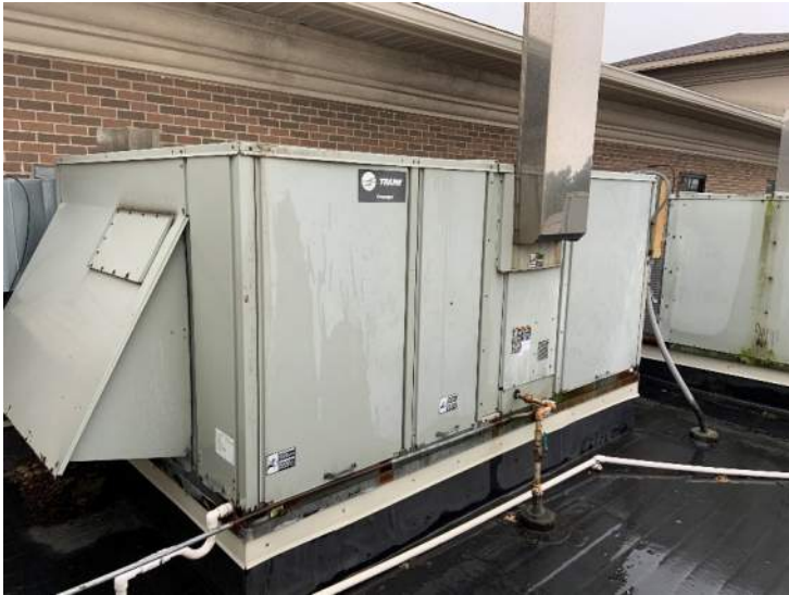
Photo 3: Rooftop Unit RTU-2
