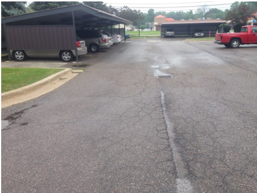
Photograph No. 6: Moderate severity fatigue cracking with crack sealing and standing water near boring B-8. View to the north.
