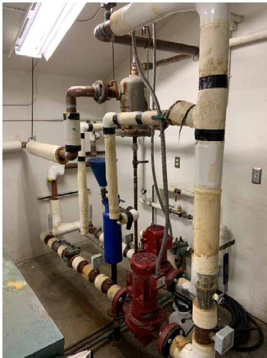
Photo 12: Hot Water Heating System Secondary Pump and Accessories
