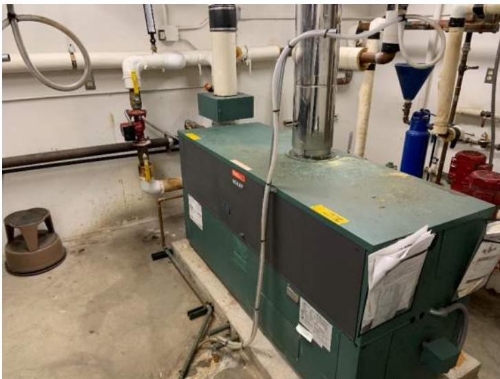
Photo 10: Hot Water Heating Boiler and Primary Pump
