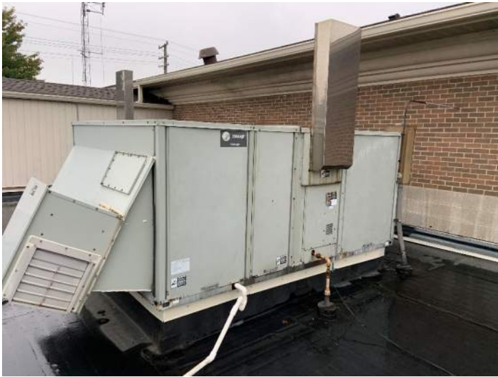
Photo 5: Rooftop Unit RTU-4
