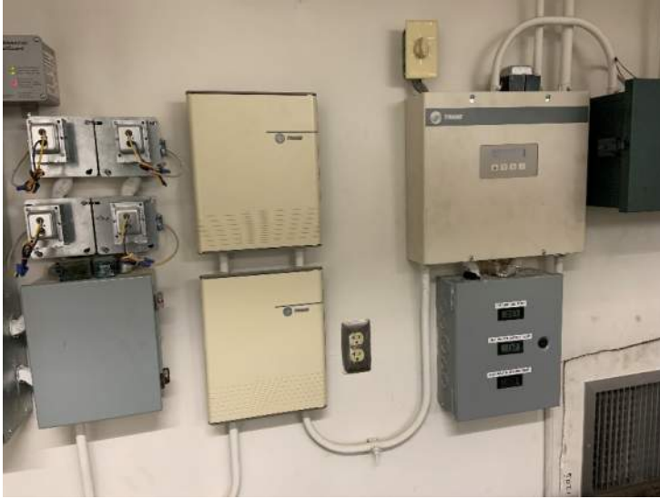
Photo 11: Boiler Control Panel and Temperature Control Panels
