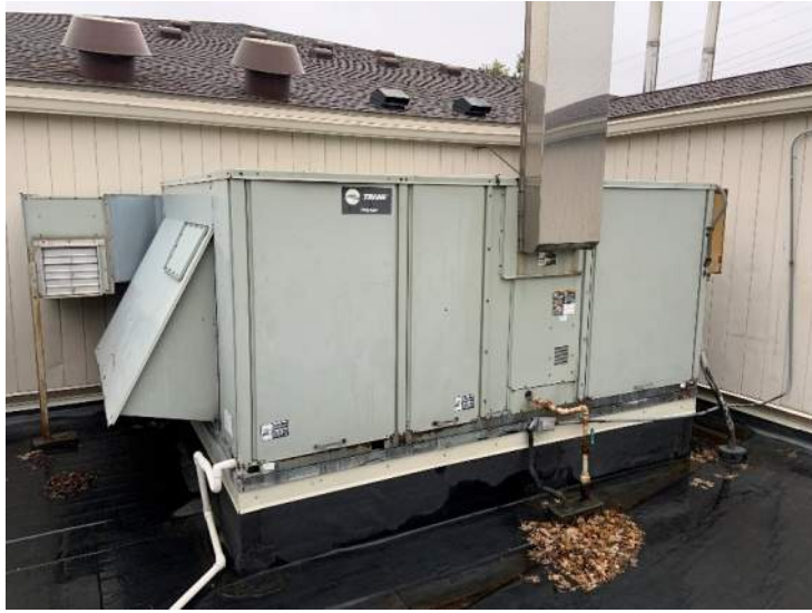
Photo 1: Rooftop Unit RTU-1
