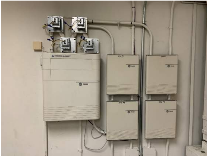
Photo 8: Temperature Control Panels
