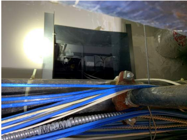
Photo 13: Air Terminal Unit above Public Safety
