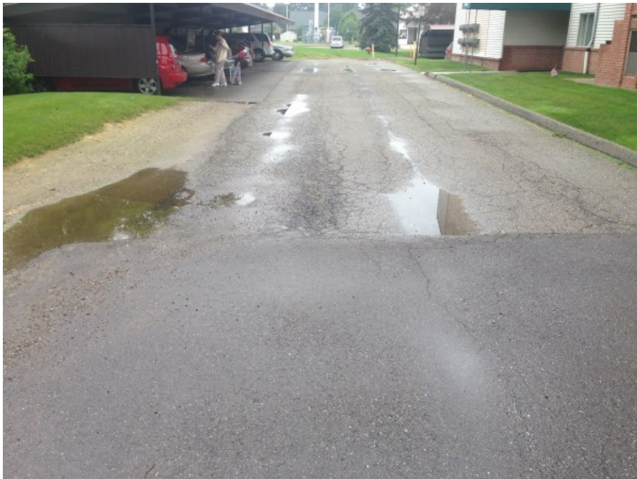
Photograph No. 4: Moderate to high severity fatigue cracking with full depth replacement patching, pavement rutting, and standing water near boring B-5. View to the west.
