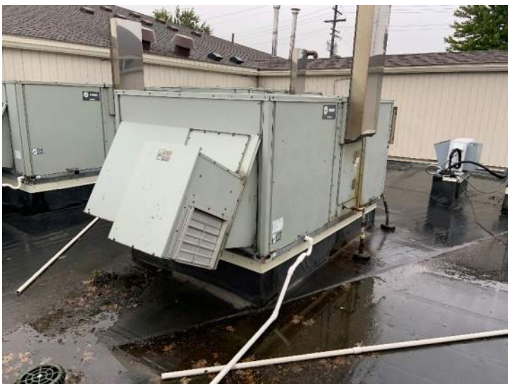
Photo 4: Rooftop Unit RTU-3
