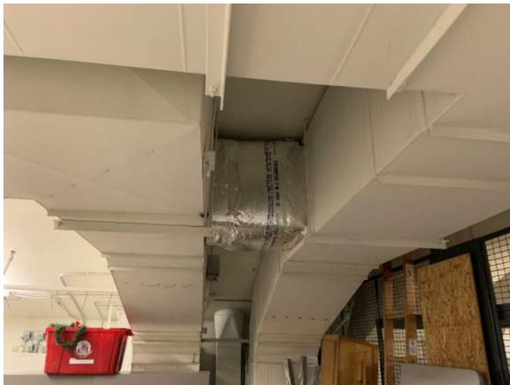
Photo 2: Bypass Damper on RTU-1
