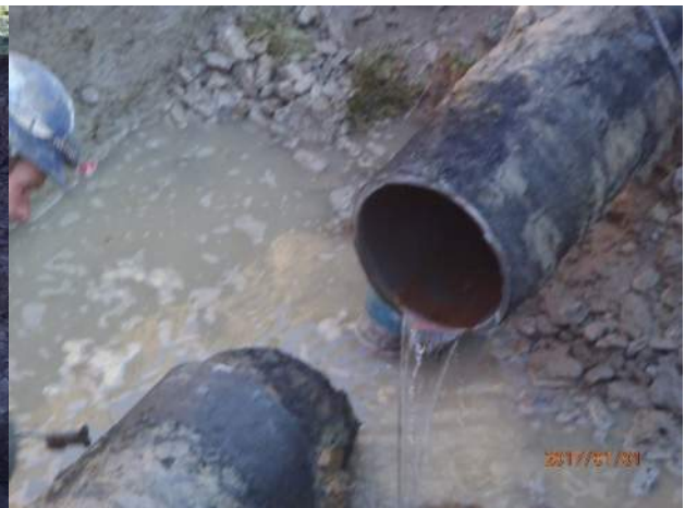
Figure 3.1-2 2016 Collapse – 2 Ft Section Cut
