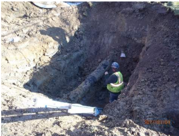
Figure 3.1-1 2016 Collapse – East of Sinkhole
