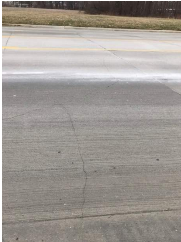
Figure 4.0-1 2019 Break – Pavement Cracking Across 15 Mile Road
