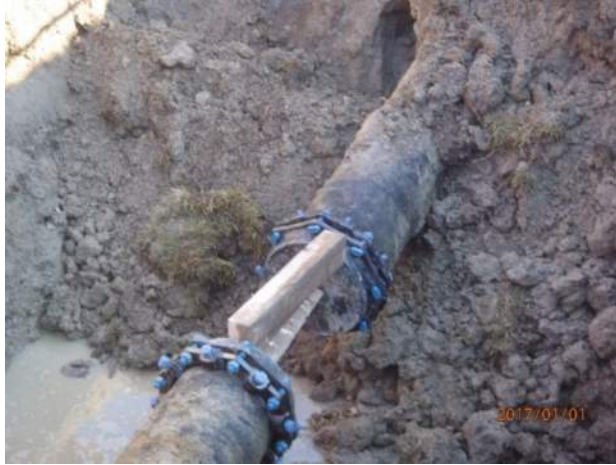
Figure 3.1-3 2016 Collapse – Both Ends Capped
