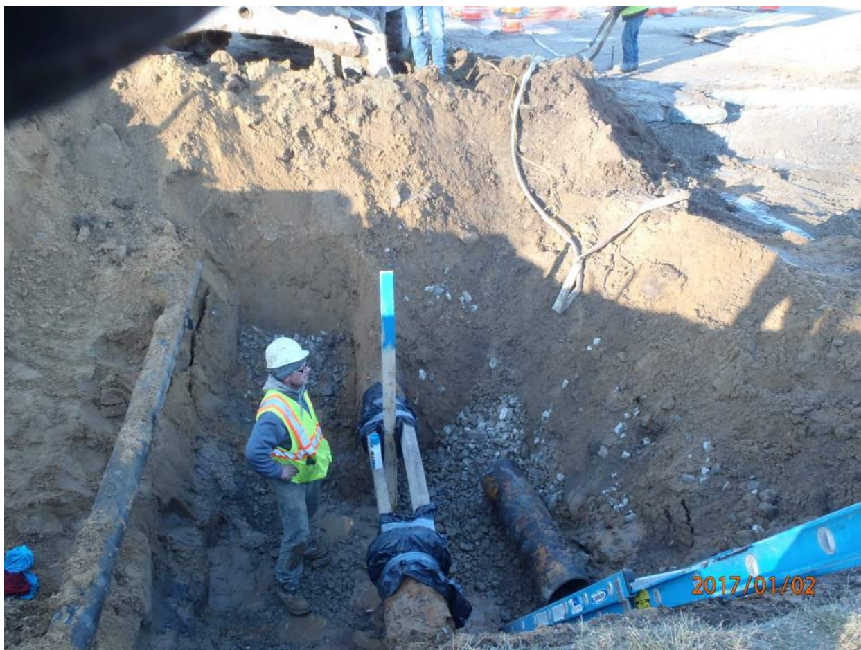
Figure 3.1-6 2016 Collapse – Location Stake
