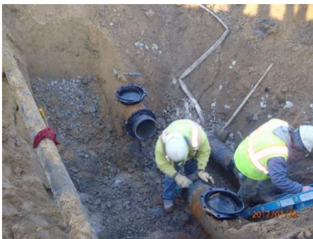
Figure 3.1-4 2016 Collapse – West of Sinkhole
